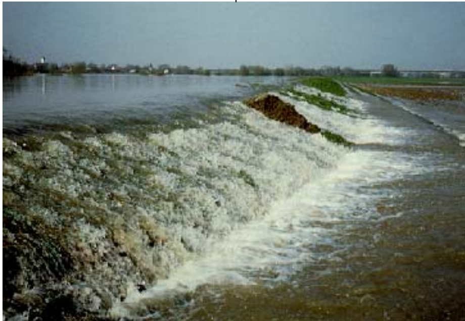
Overtopped Danube dike during flood in 1994 (Source: WWA Deggendorf)
