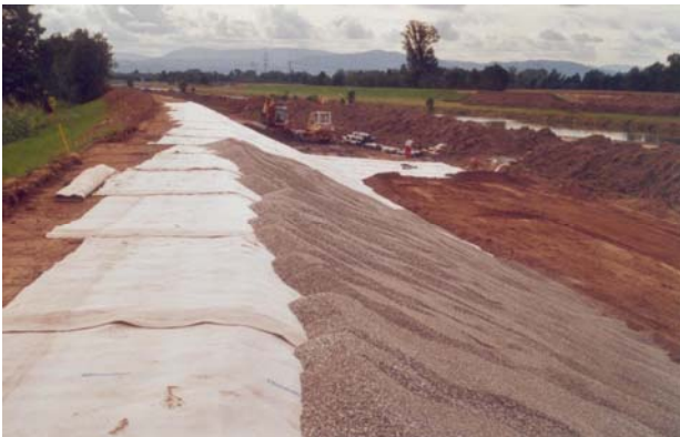
Figure 2. Rehabilitation of dike slope along the Kinzig River (2001): covering of the GCL Bentofix with gravel as an "animal deterring" cover layer (right)
