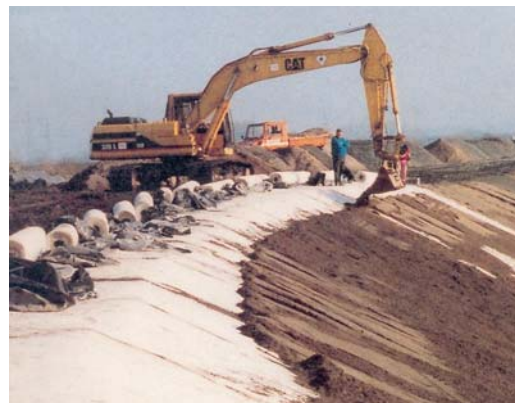
Figure 3. Lippe River dike rehabilitation (1994): installation of Bentofix GCL as a sealing layer
